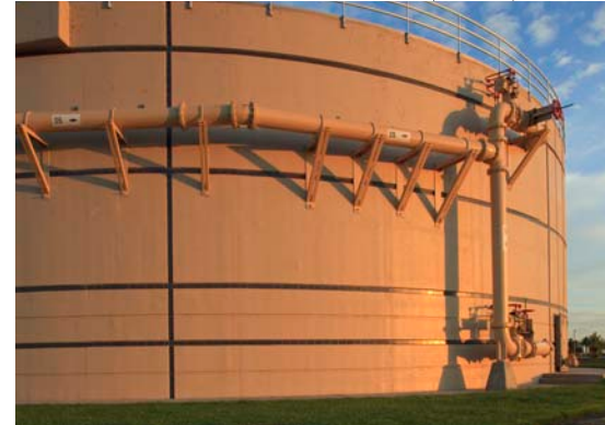
Anaerobic Digester – Fresno, CA
