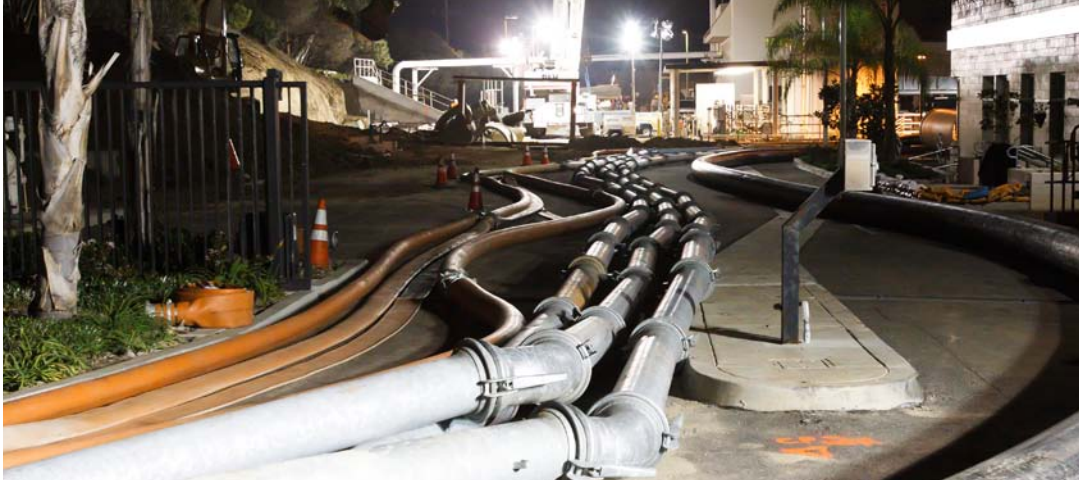
Bypass piping – Encina
