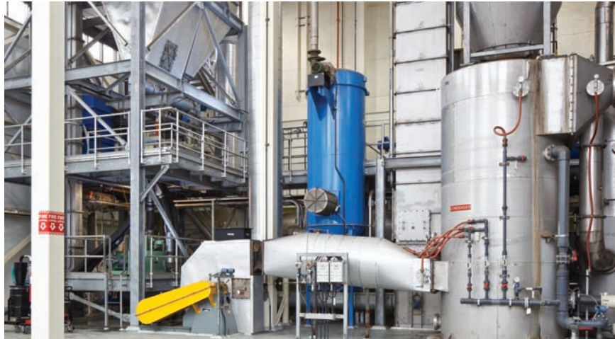
Encina Water Pollution Control Facility – Pelletizer
