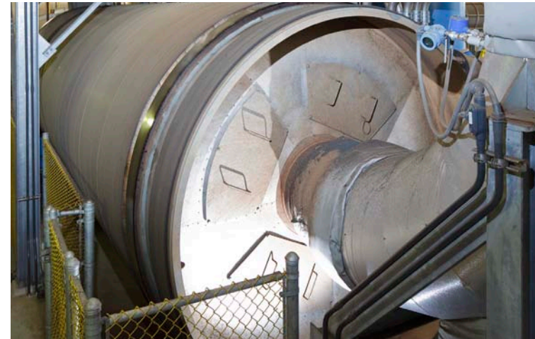
Encina Water Pollution Control Facility – Dryer
