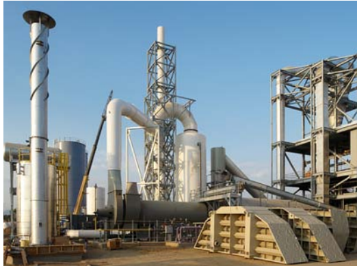
Slurry Carb Facility, Enertech – Rialto, CA
