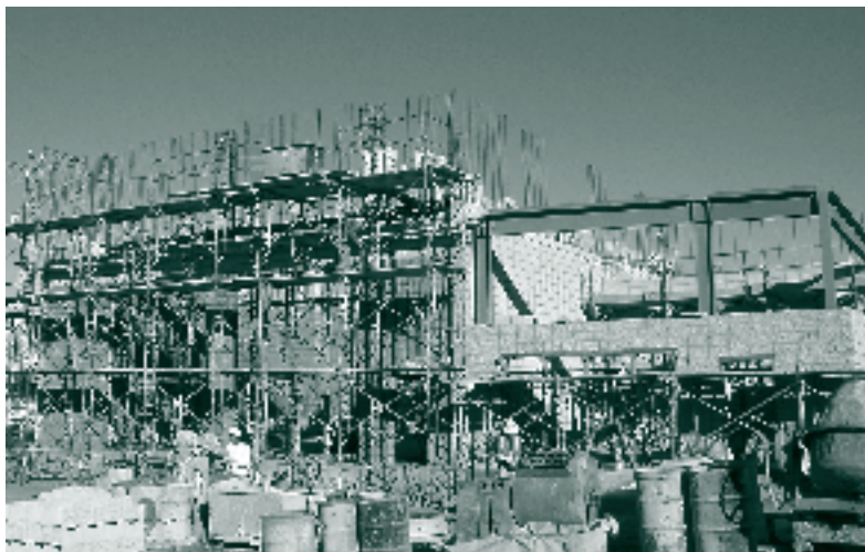
Henry J. Mills Treatment Plant chlorine facility
